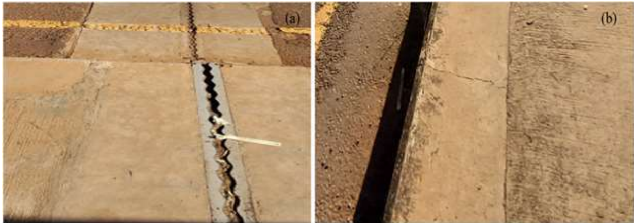
Figure 5: Photos of defects for Kikwete Bridge (a) blockage by siltation and (b) cracks on a walkway
